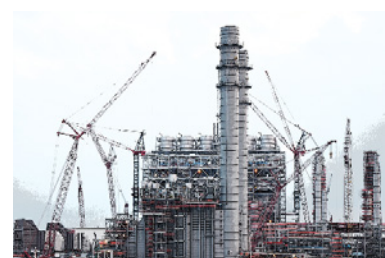
Mississippi Power's Kemper IGCC project with CO 2 capture (Source: www.biggerpieforum.org )
